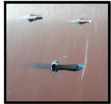
View from inside the return air duct demonstrating how the probe protrudes through the sheet metal into the air stream.
